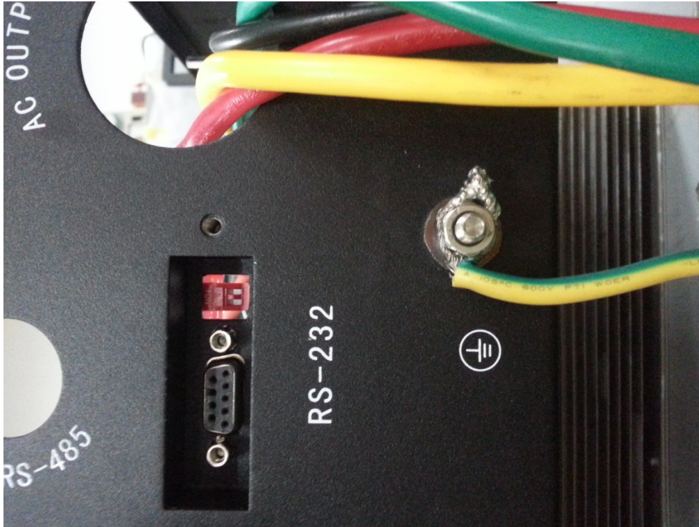
Earthing terminal of the unit
